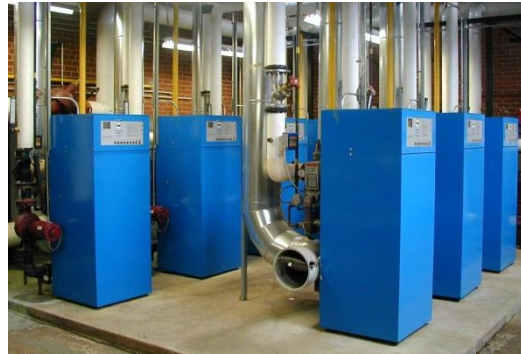
Heating & DHW Boilers 14" W.C.
