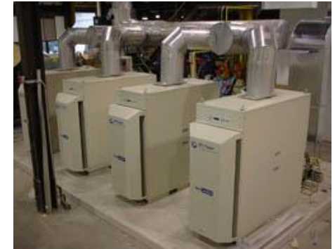
Power Generation 1-3 PSI
